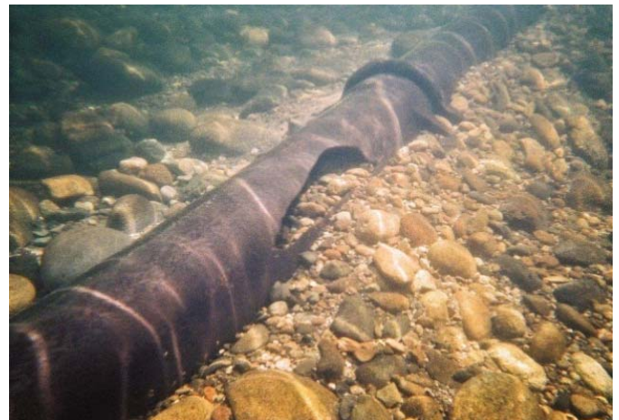
A de-commissioned watermain in the Kettle River, which was originally buried in the riverbed
